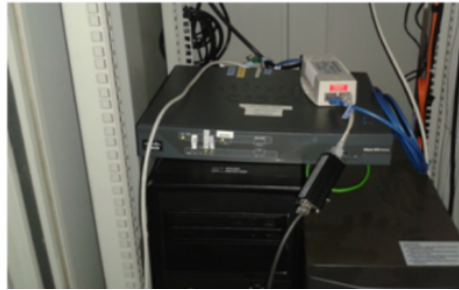
TVWS LAN Equipment: PEO Injector, Router and Server
