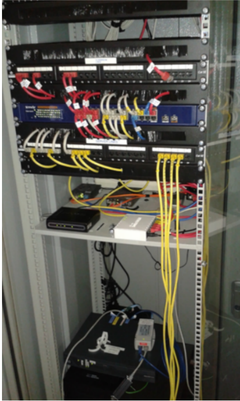
School LAN Equipment
